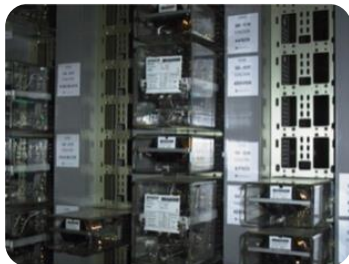
Track Circuit Test Setup
