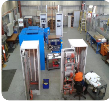
Electrical Substation Workshop
