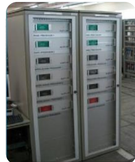
SSI Test Rack
