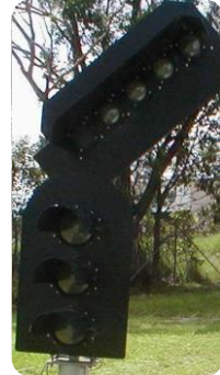
Junction Route Indicator LED Signal
